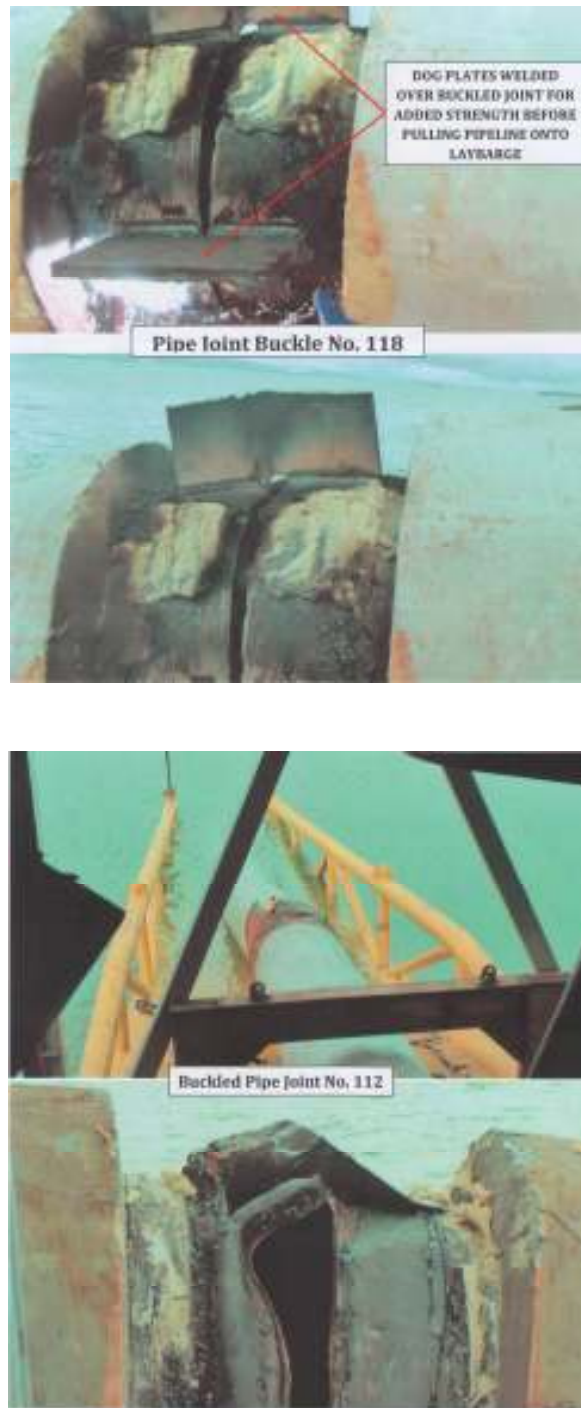
Rajah 8: Pipe buckling.
