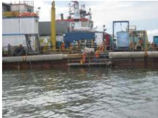
Rajah 13: Tie-in of pipes laid by laybarge and laybarge shore pull method near Labuan shore.
